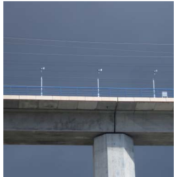
Crosswind detection station installed on a viaduct.
